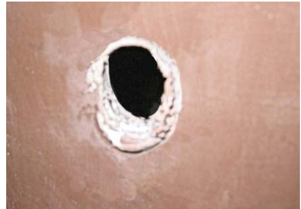
Bolt Hole Elongation - exterior
